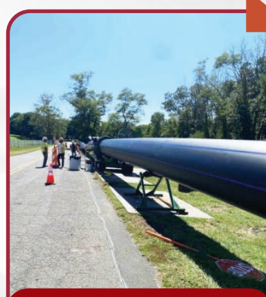
North-South Transmission Main improvements enhance operational flexibility.
