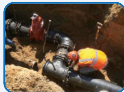
District personnel install water main at the intersection of Haypath Rd and Lent Dr.
